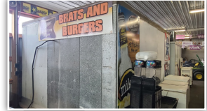
WALK-IN COOLER & FREEZER
